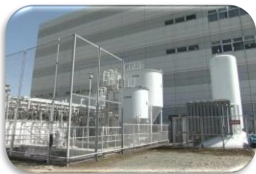
Effluent treatment facility (Sayama Plant)
